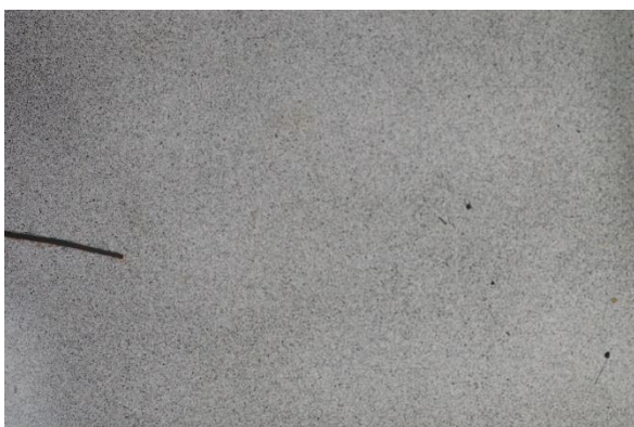
Figure 10. Crack/defect the area
