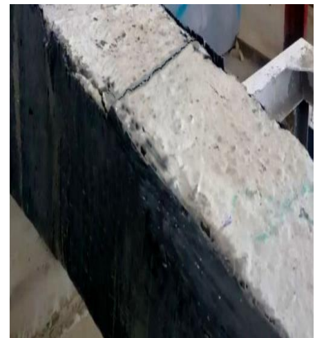
d) failure crack from the top
