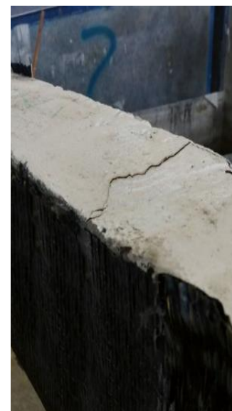
d) failure crack from the top
