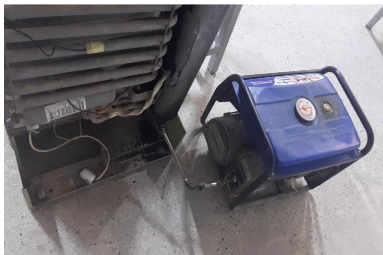
Figure 2. The process of connecting the pipe between the generator and the refrigerator
